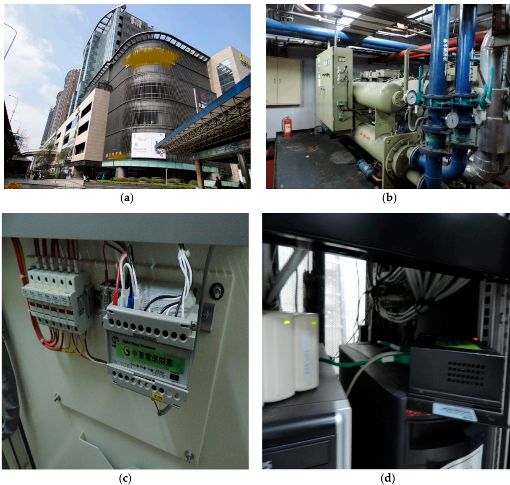
Figure 1. A real test site for presenting artificial intelligence (AI)-assisted heating ventilation and air conditioning (HVAC) control performances. (a) The case study facility; (b) the chiller system including 6 chillers installed in the building; (c) a power meter for measuring the energy consumption; (d) a networked temperature/humidity sensor module for detecting the necessary parameters for the HVAC control.
